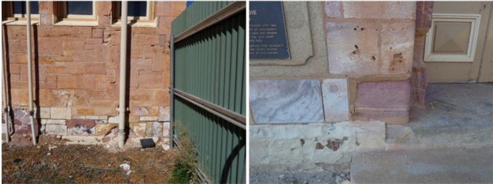
Figures: External stone fretting and mortar failure
