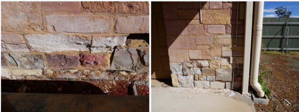
Figures: External stone fretting and mortar failure
