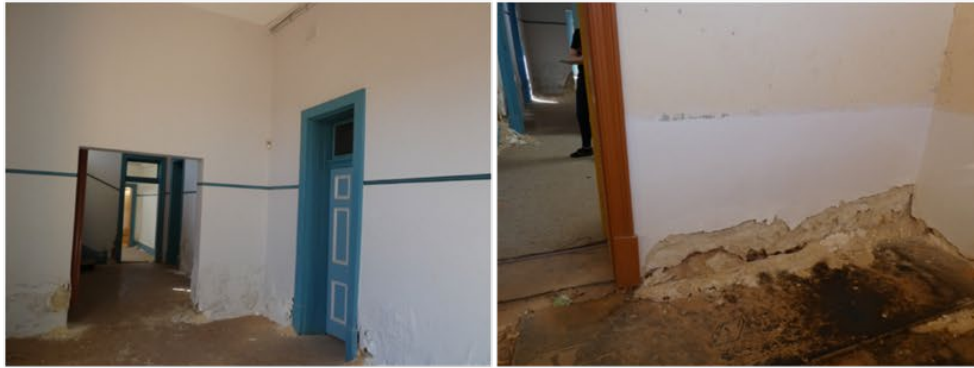
Figures: Interior rising damp and salt attack with failing render (worst affected areas)
