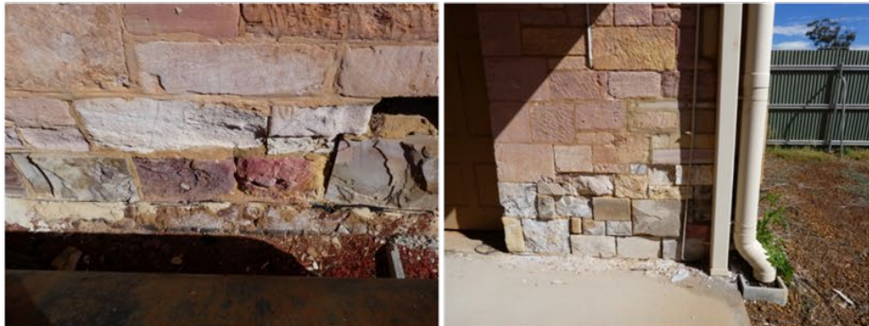
Figures: External stone fretting and mortar failure
