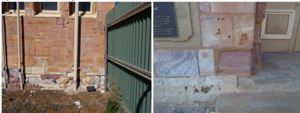
Figures: External stone fretting and mortar failure
