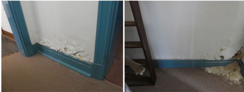
Figures: Interior rising damp and salt attack with failing render (less affected areas)
