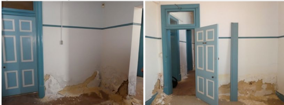
Figures: Interior rising damp and salt attack with failing render (worst affected areas)
